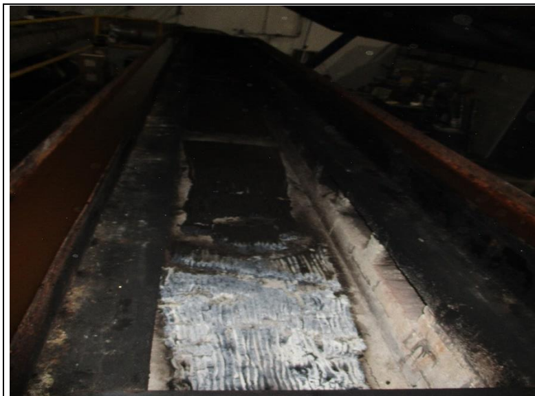
Photo No. 2 Post Test
